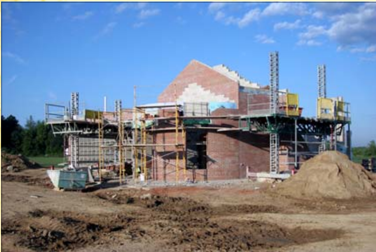
St. John Cemetery Richfield and Oak Rd. Davison, Michigan r Mausoleum Construction Summer 2006
